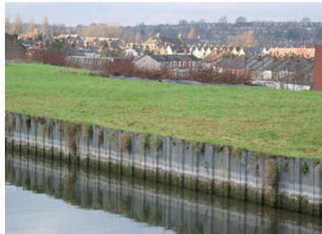
Along the northern edge of the site to the New River has a utilitarian character
