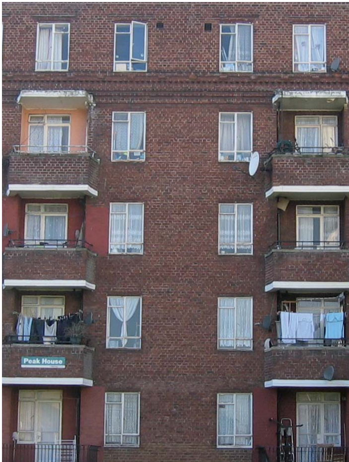
Externally the design of blocks lack quality and character
