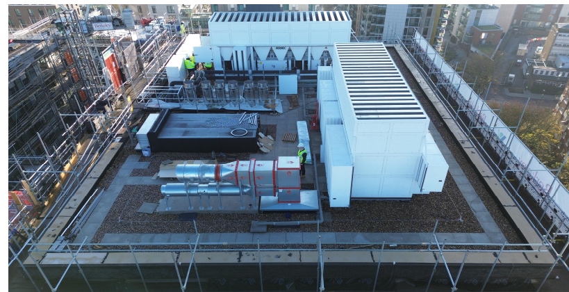
Air Source Heat Pumps
