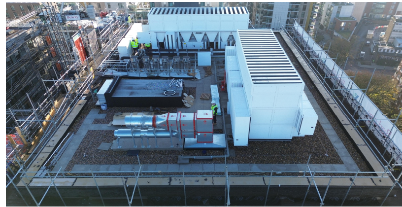
Air Source Heat Pumps
